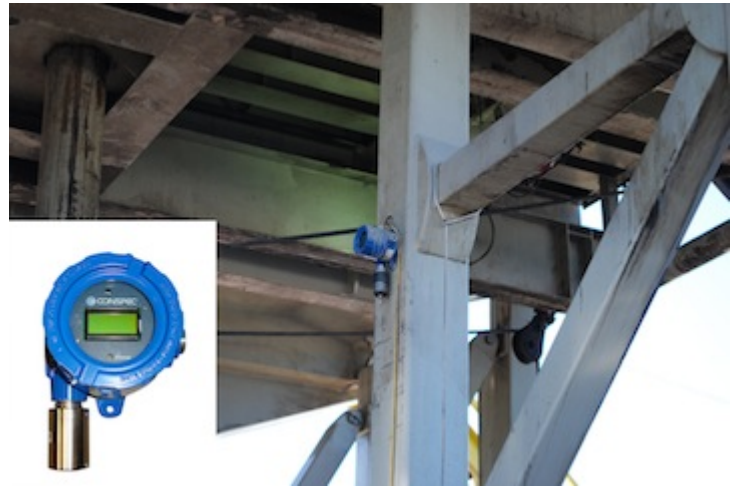
CX Series Monitor installed on rig.
