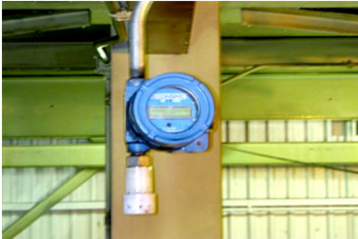
fig. 5 - Typical CO monitor installed along a belt head drive location. Note the white cap on the sensor head. This is the splash guard used to prevent wash-down work from loading the sensor with water.
