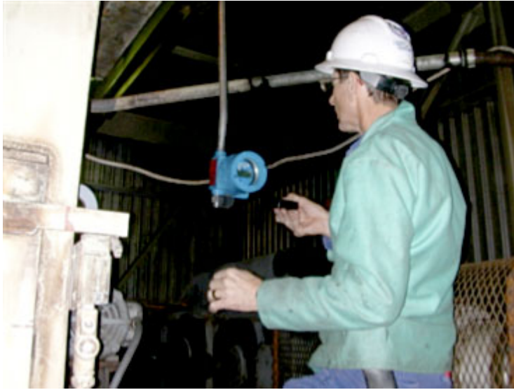
fig. 4 - A CO monitor undergoing calibration during initial installation at the top of the conveyor structure
