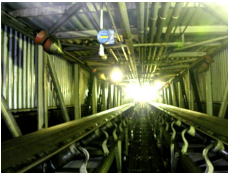
fig. 6 - Looking down the main conveyor structure. A CO monitor located above and left of center. Two conveyor belts on either side, redundant to minimize the potential of shutting down the plant if a single conveyor shuts down.
