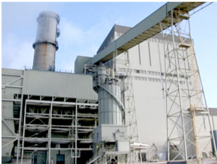
fig. 7 - This is the view of the main conveyor as it heads into the power plant building, which is about 13 stories high
